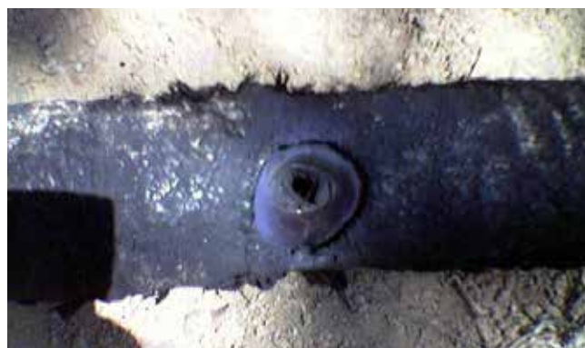
➤ Cable Fault in a 132 kV PILC cable
